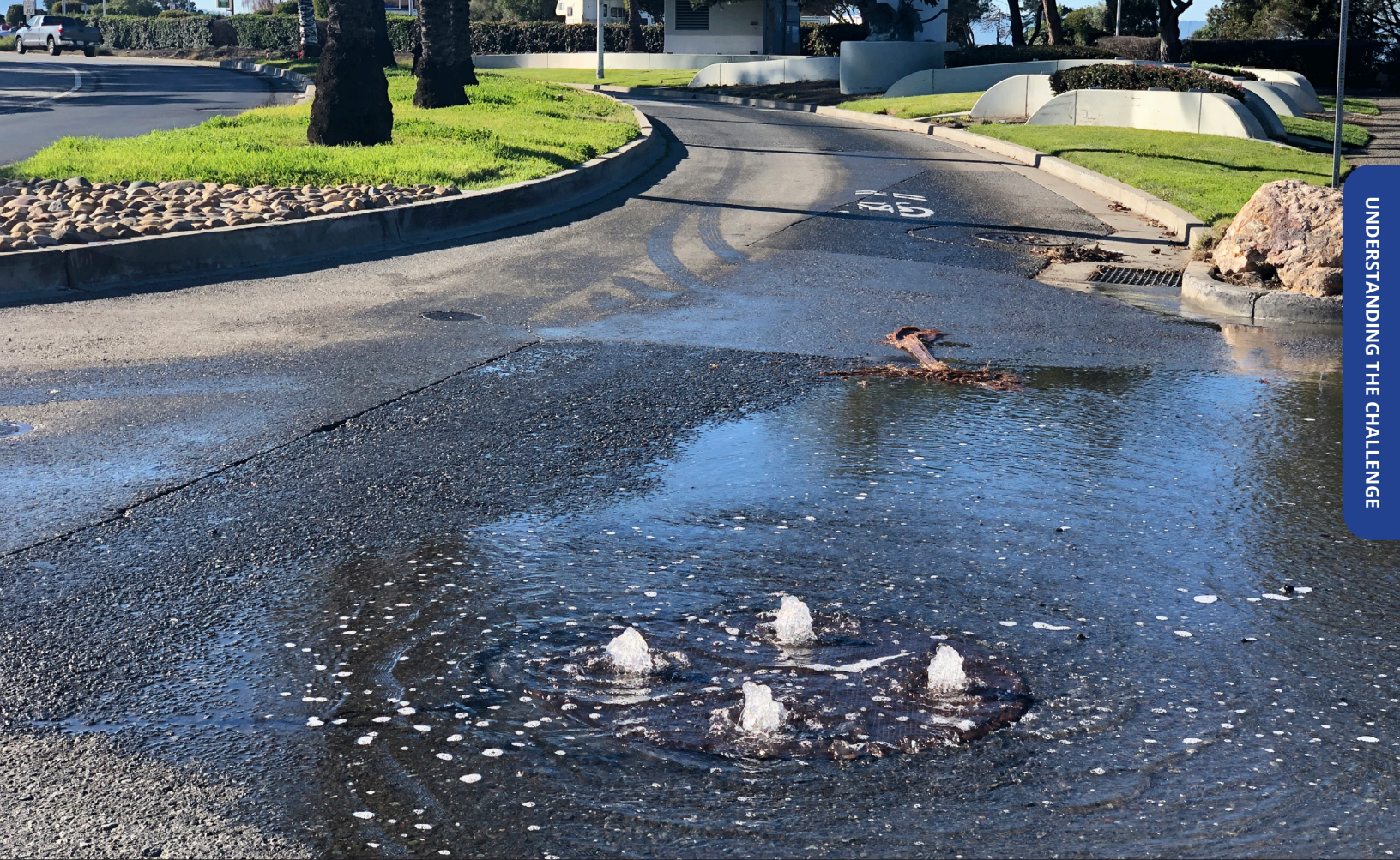
During king tides in January 2022, groundwater infiltrated into the City of San Leandro storm sewers along Marina Boulevard, percolating out of manholes and flooding roadways. Photo Credit: Kristina Hill
